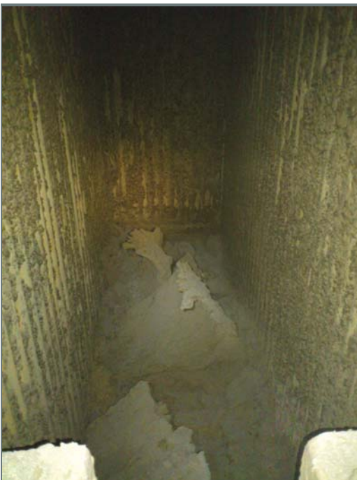
Before Shock Pulse Generator installed
