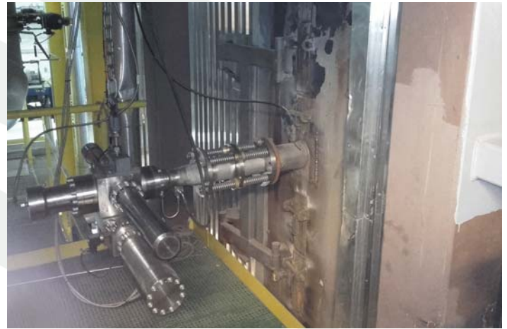
Shock Pulse Generator installed at Sarpsborg
