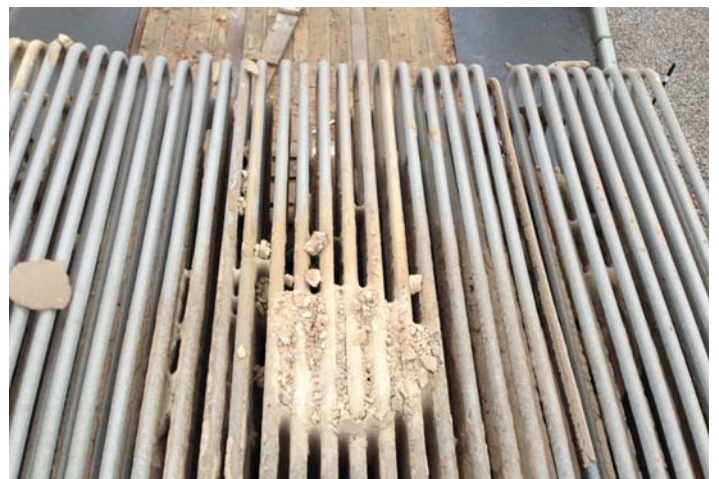
After: Tubes removed from the boiler after installing a Shock Pulse Generator – much cleaner than tubes in photo to left of page
