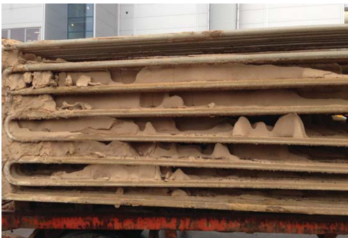
Before: Tubes removed from the boiler before installing the Shock Pulse Generator
